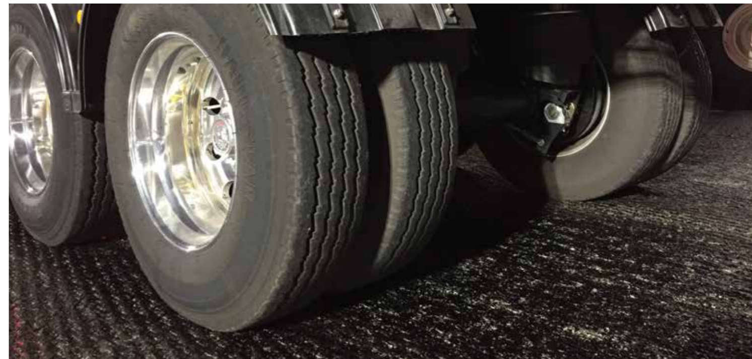
Top: Figure 2 – Application of tack coat Bottom: Figure 3 – Trackless Tack coats – The emulsion is not picked up by truck tyres
