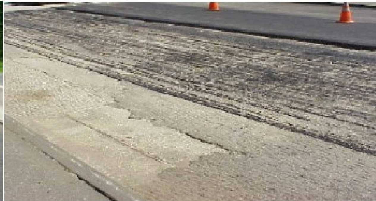
Figure 2. Poor tack coat coverage.
